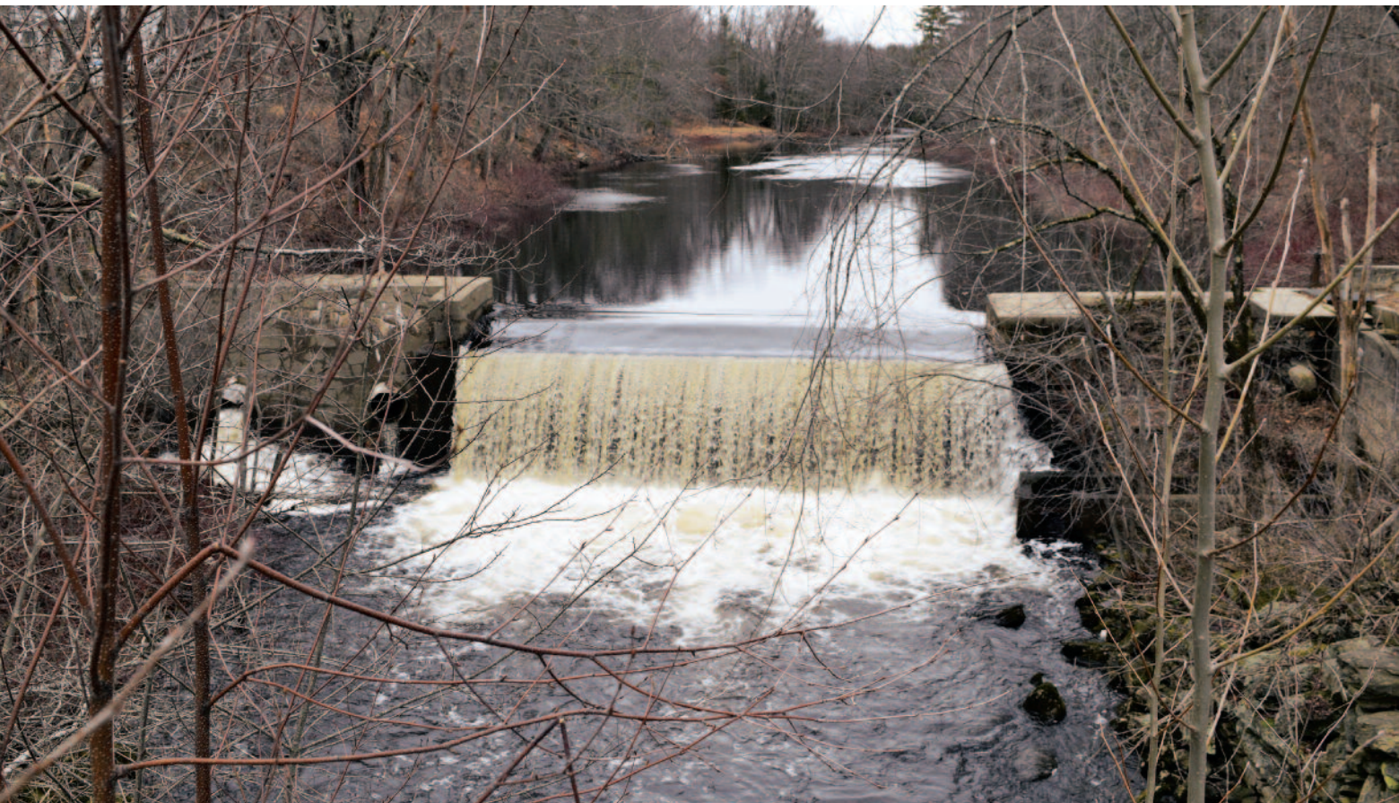
The Head Tide Dam, built in 1916, is cherished by townspeople but in dire need of repairs, thus offering an opportunity to improve fish passage (top). ASF is working with local partner the Midcoast Conservancy to remove the Coopers Mills Dam on the Sheepscot River (above).
