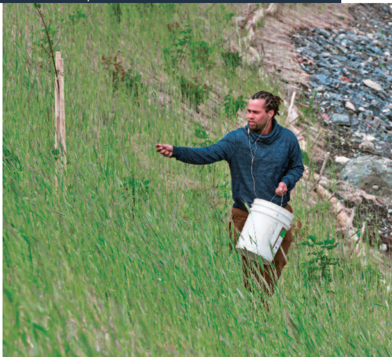
Final touches: Wild seeds are spread to strengthen the banks of the bypass area.
